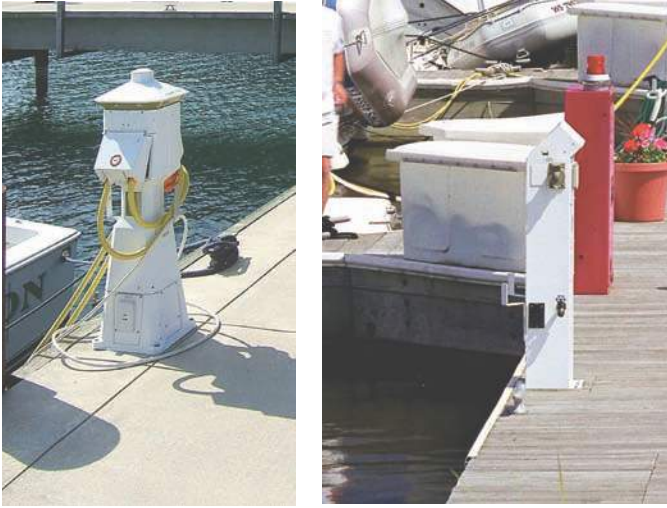
Typical dockside utility centers
