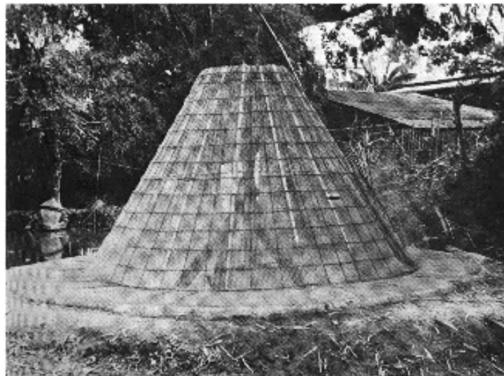
Figure 2.10 The frame is completed with one layer of wire mesh on the outside surface and one on the inside. Mesh, reinforcing rods, and struts are fastened together with short lengths of wire threaded through the wall and back and twist-tied with pliers. ( Applied Scientific Research Corporation of Thailand )
