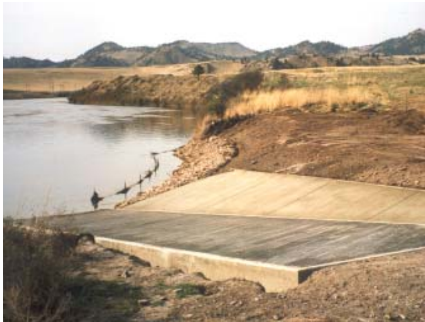
Photo 8A, 8B: An elliptical concrete ramp was installed at Wolf Creek, on the Missouri River, to reinforce the bank and provide a loading area for paddlers in a way that helped mitigate erosion
