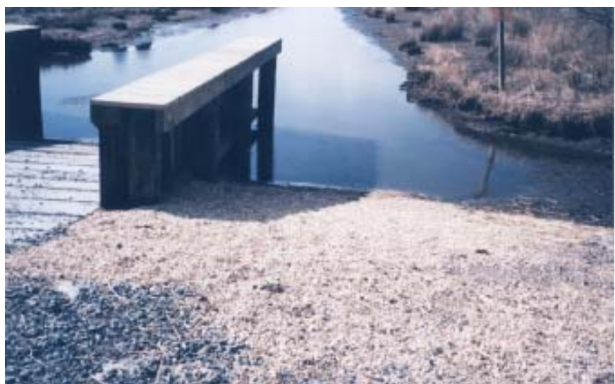
Photos 11B: Geocell material anchored with pea gravel offers low-impact access while helping to stabilize an eroding bank
