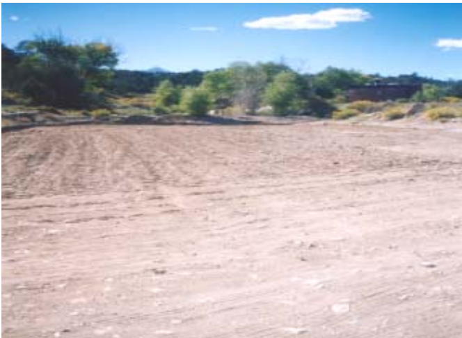
Photo 8L: Drainage area adjacent to launch site carries heavy flows during spring runoff and causes scouring
