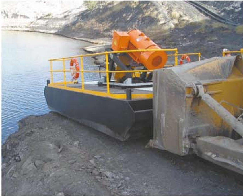
Above: Using a dozer to launch the pontoon pump unit down an access ramp.
